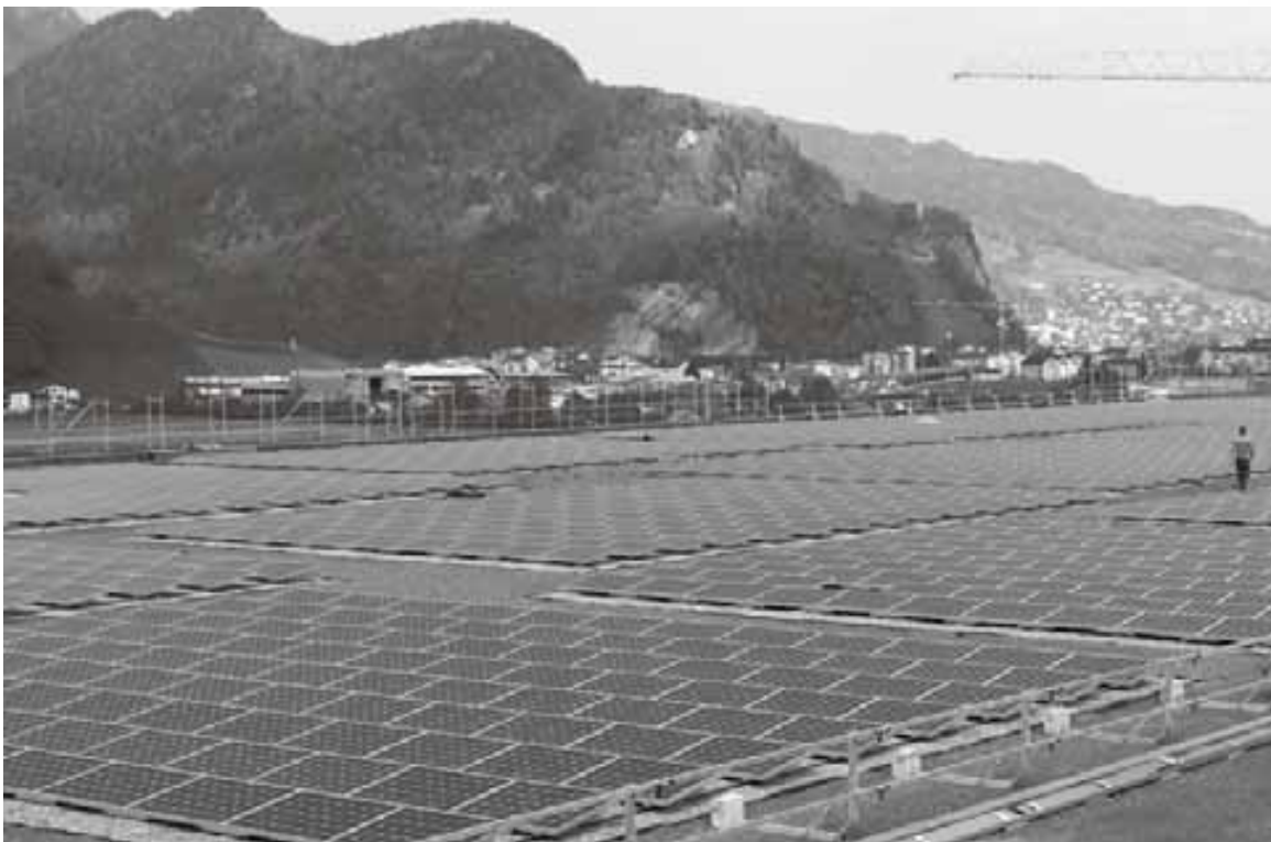
Photovoltaik-Anlage L nderpark Stans
